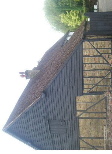
Fig 5.18: Old Mill House- timber framed barn with stained weather boarding
